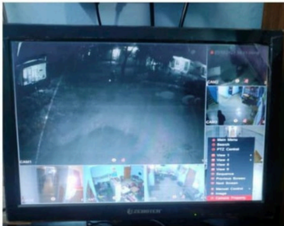
CCTV surveillance (Girls' Hostel)
