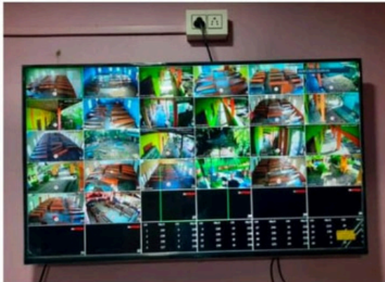
CCTV surveillance (College Campus)
